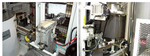
Detailed study of processes lead to find optimum solutions to all problems
